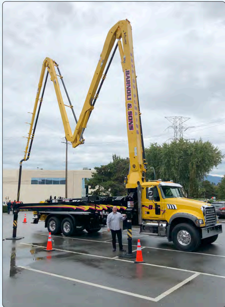
BCCSA's Lui Garcea stands near concrete boom pump at CCPO launch event.
